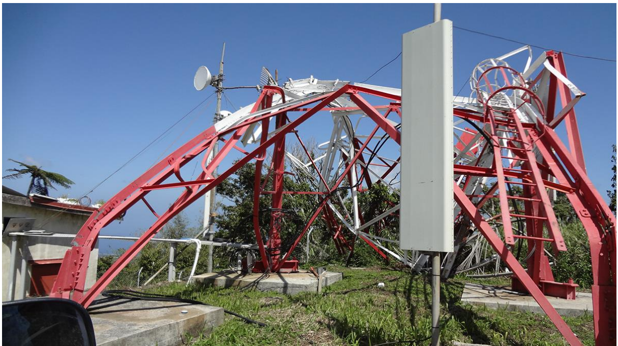
----- TC PAM Destroyed Telecom Tower in Vanuatu
